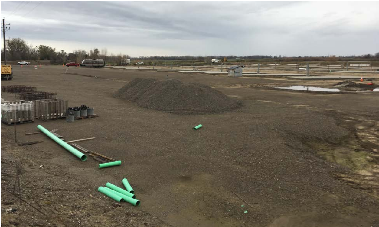
Figure 2. Site photograph taken by U.S. Army Corps of Engineers biologist on February 25, 2019.
