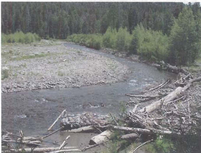
Figure 1 Looking upstream from bridge at eroded bank
