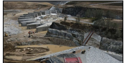
Photo shows aerial visual overlooking the Labyrinth Weir and Main Dam Control Tower.
