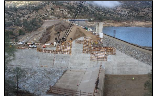
Improvements to the existing service spillway at Isabella Lake, looking west from between the dams toward SR155. (Photo: U.S. Army Corps of Engineers)
