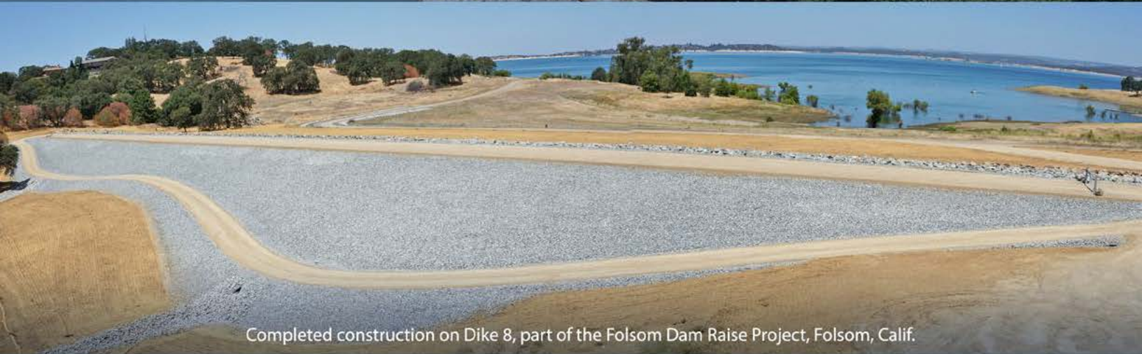
Construction of Sacramento River East Levee improvements, part of the American River Common Features (ARCF) Water Resources Development Act (WRDA) 2016 Project.
